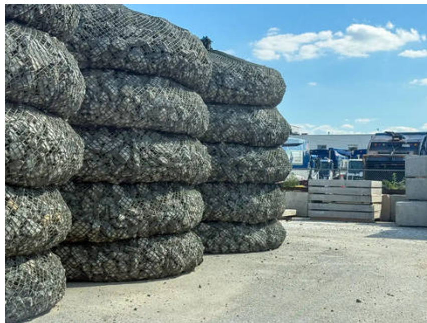
Fig. 31 Rock bags protect underwater cables and can be lifted for access. Photo: Tom Fox.
